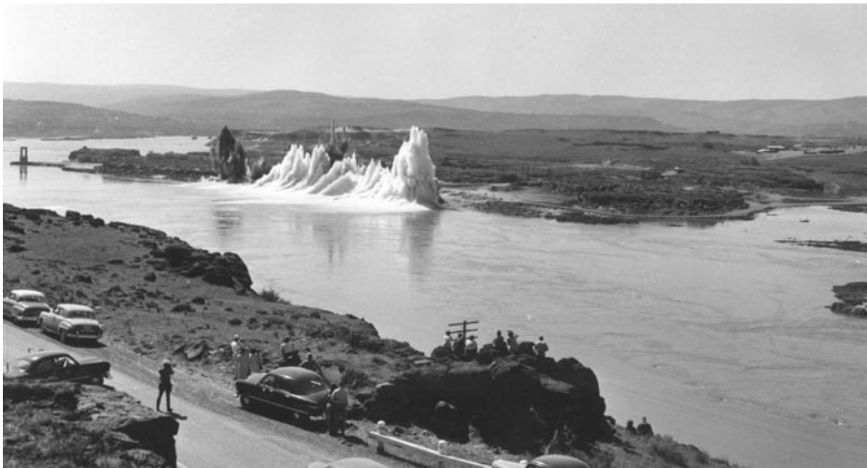
Blasting for The Dalles Dam, 1950s. Image courtesy of the Army Corps of Engineers
